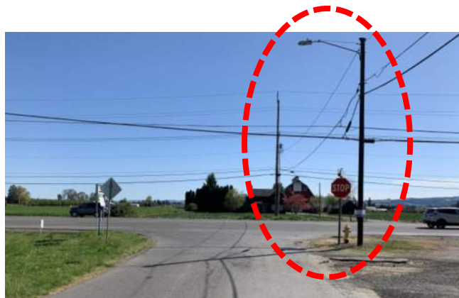
Luminaire oriented towards side street
