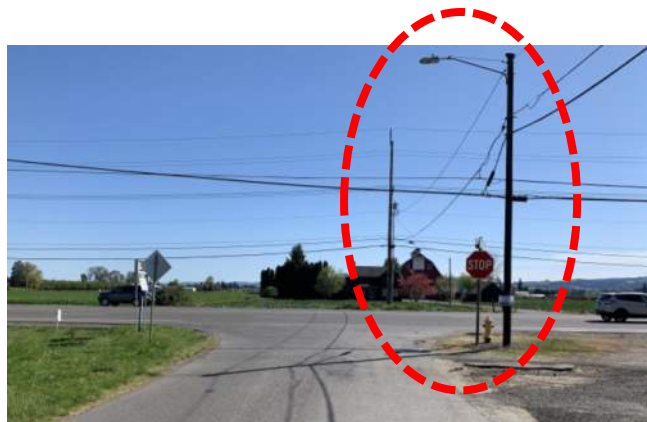
Luminaire oriented towards side street
