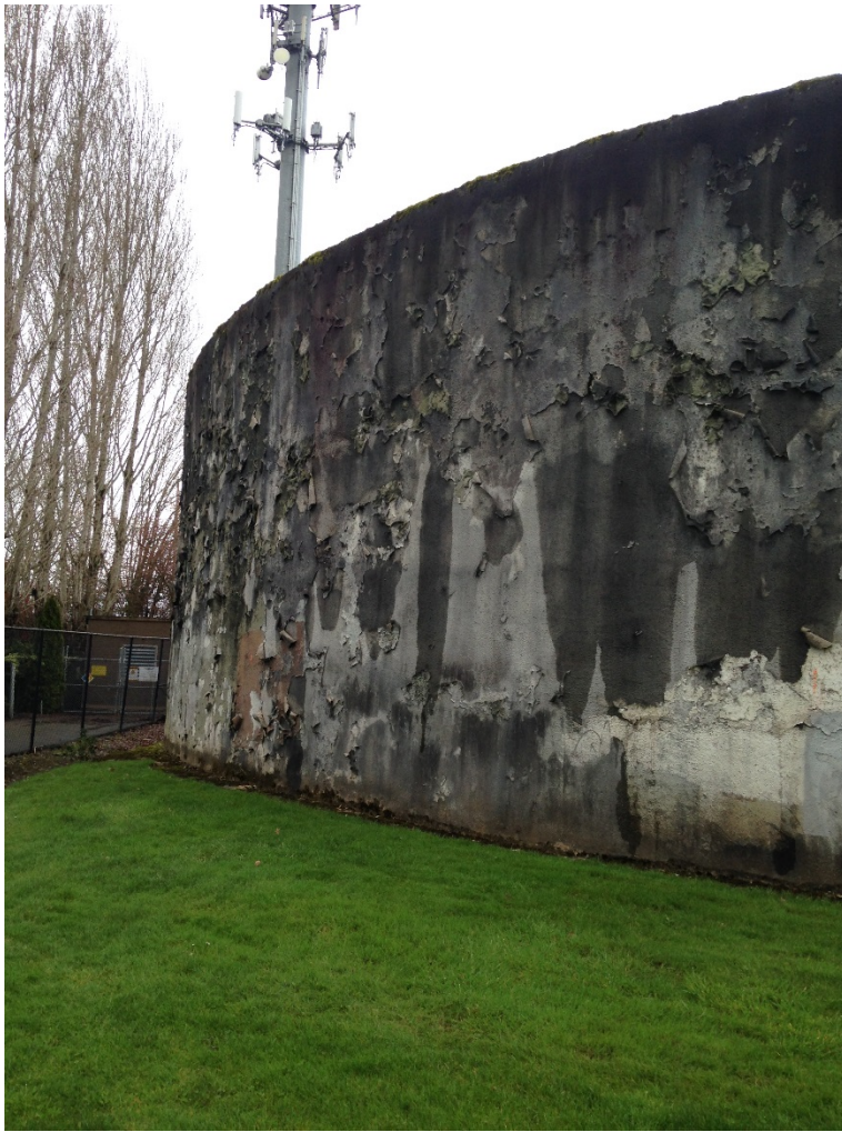
Figure 2-2. Photo of Existing Reservoir Tank Showing Failing Coating
